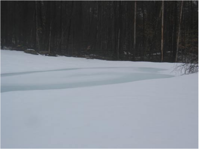
Photograph of same wet pond – Town of Hague subdivision taken on March 20, 2008. Note that there is no freeboard on the standpipe above the ice resulting in direct discharge of runoff without management or treatment.
