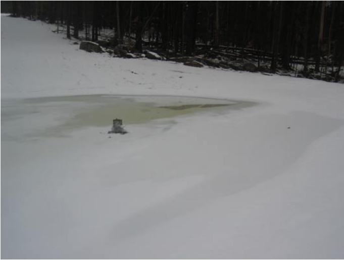
Photograph of wet pond - Town of Hague subdivision taken on January 30, 2008. Note the freeboard height of the standpipe above the ice elevation.
